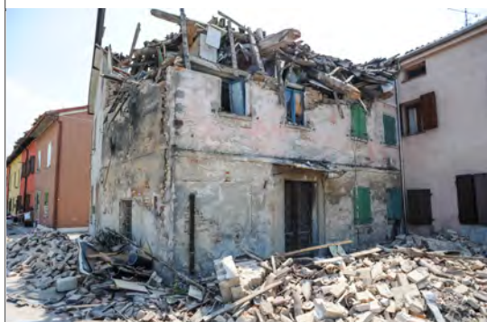
Earthquake damage in Italy 2016
